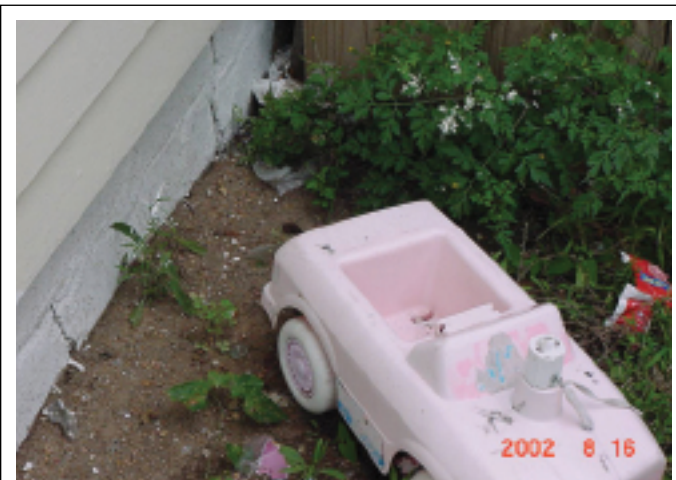
FIGURE 5.9 Soil lead hazard at dripline
