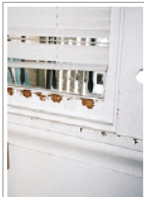
FIGURE 5.8 Chewable surface: teeth marks on window sill.
