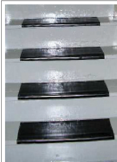
FIGURE 5.6b Friction hazard on stairs post-treatment.
