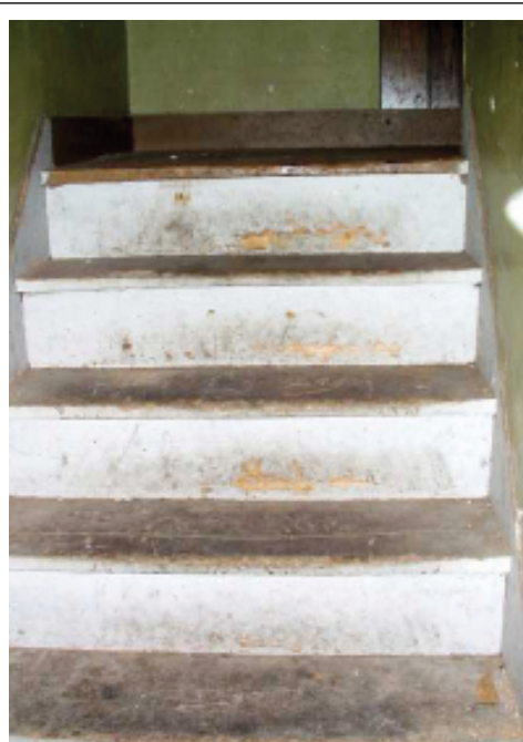
FIGURE 5.6a Friction hazard on stairs pre-treatment.
